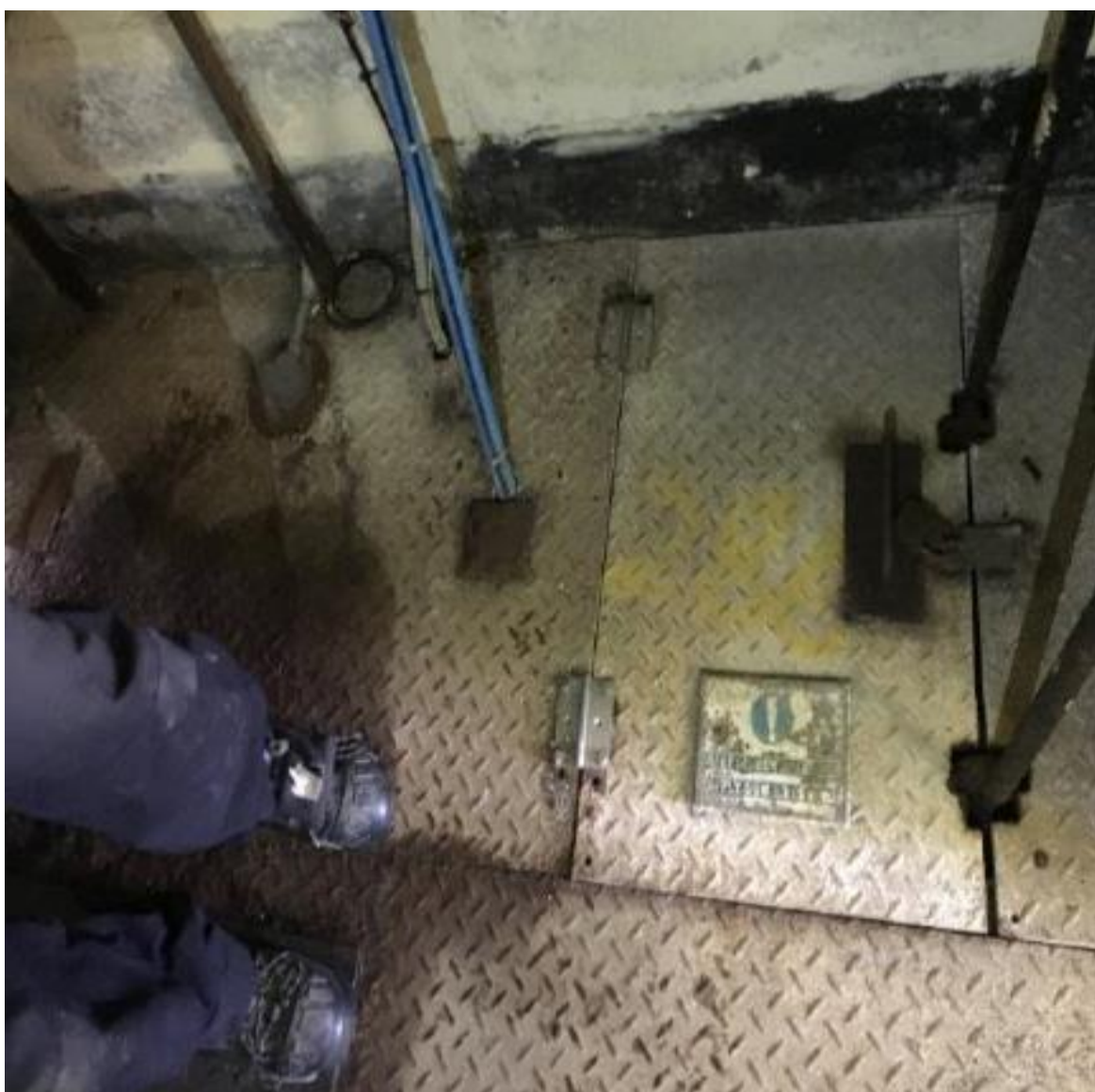
Figure 7: Poor integrity of sample hatch at United Utilities Runcorn service reservoir
