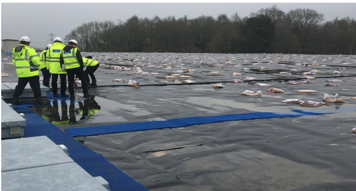
Figure 5: Rownhams Reservoir. Temporary Cover.
