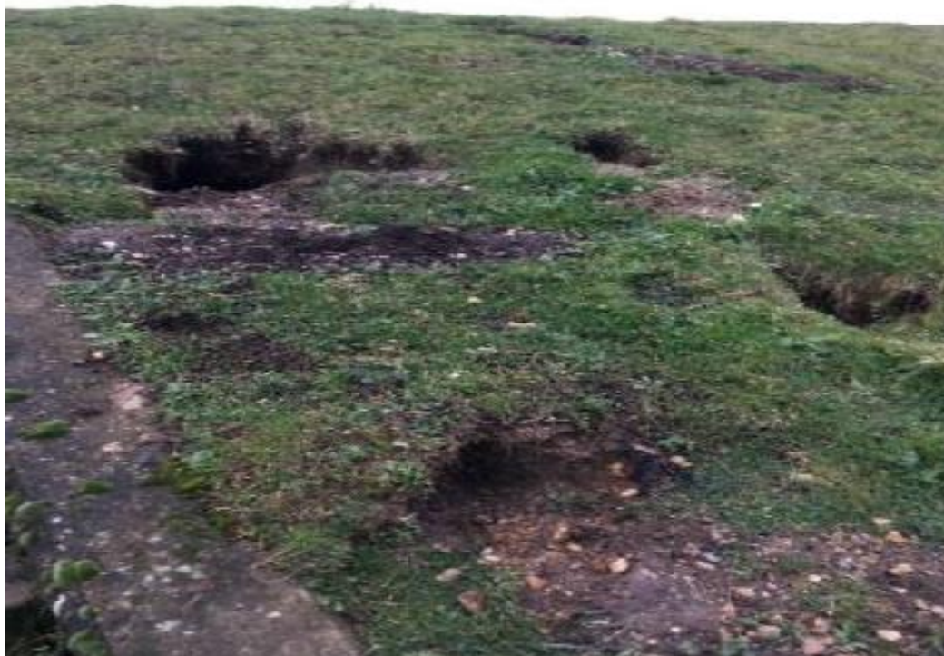
Figure 6: Jack's Hill SR – Vermin burrows into the embankment
